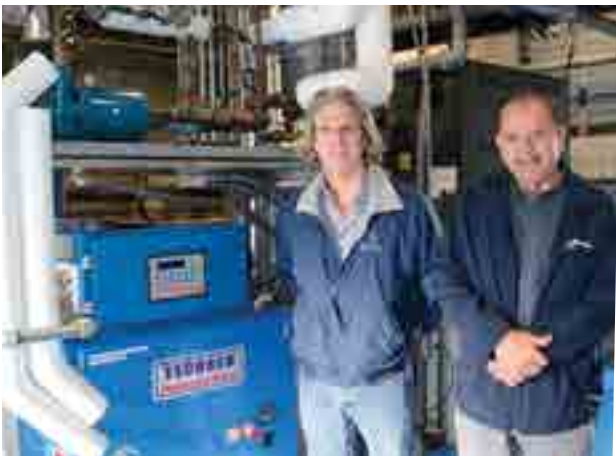
Ron Miller, Bellarmine's CFO, and Quirino Arias, Director of Facilities, with the school's new co-generator.
